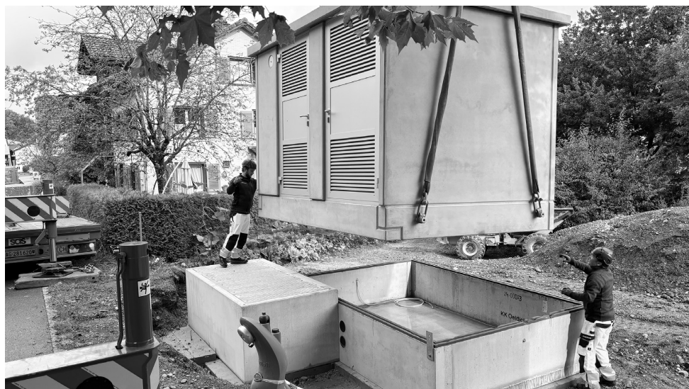
Transformatorstation Traber Bichelsee
